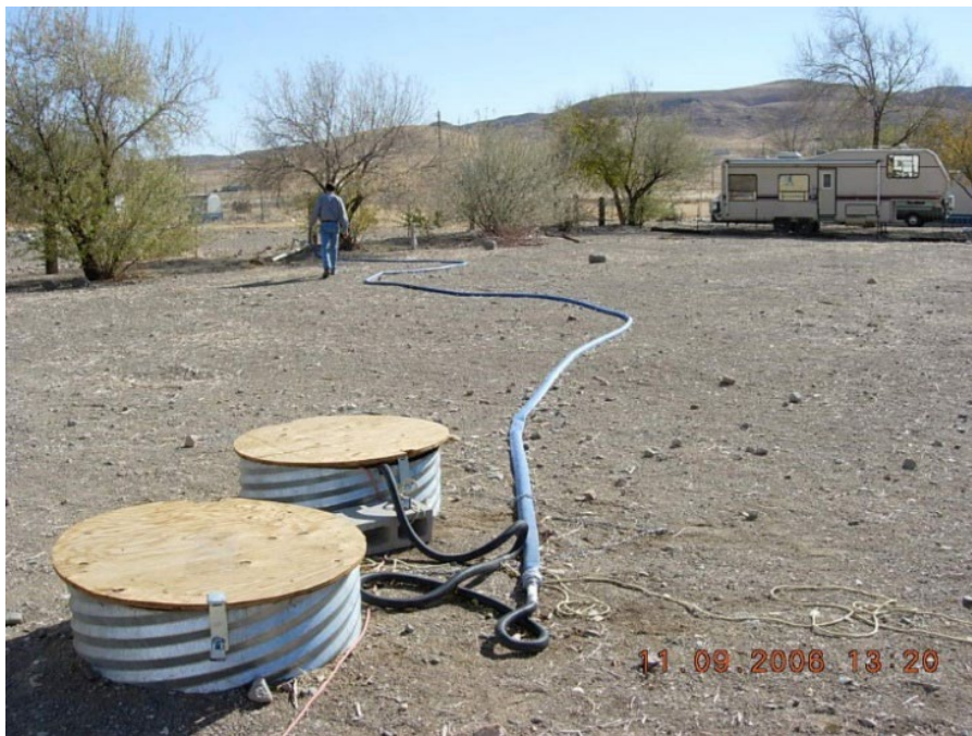
Fig. 2 – Example (unauthorized bypass of effluent)
