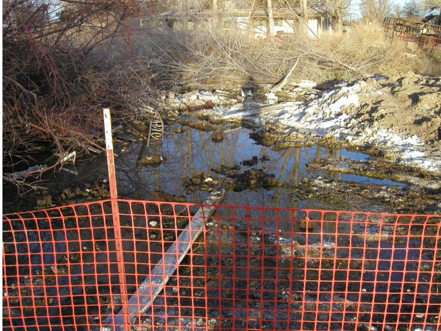
Fig. 1 – Example (failed leach field)
